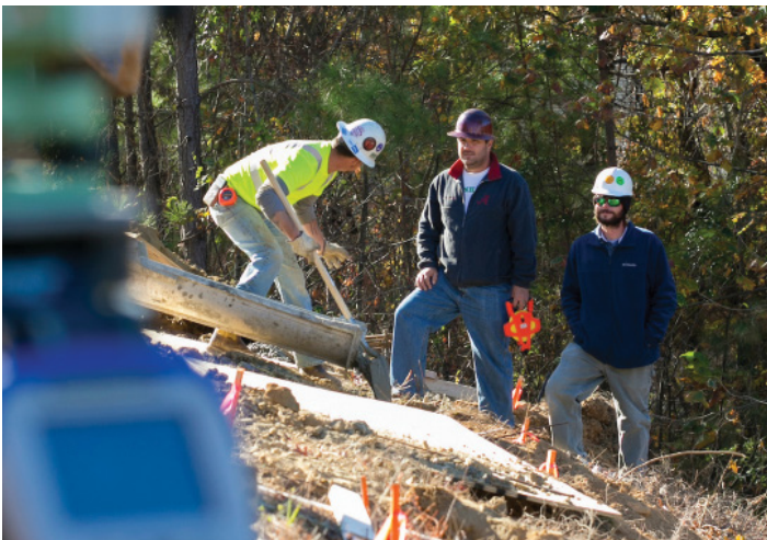
Workers prepare to pour concrete pilings for a new chilled water plant (all photos).
